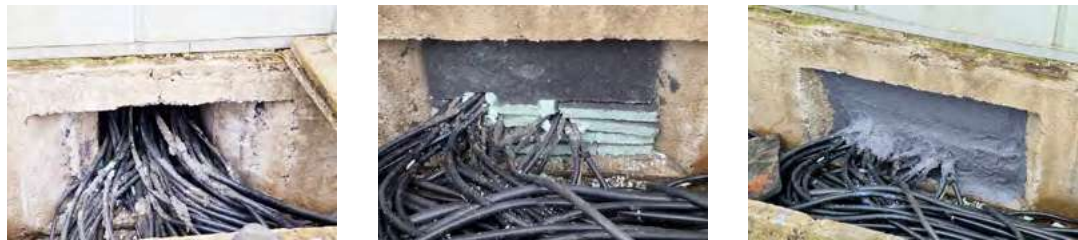
Close off a cable pathway with rodent-proof panels and PFP sealant
